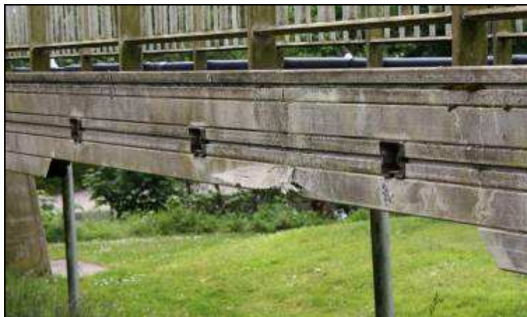
(a) Location of the damage (June 2008)
