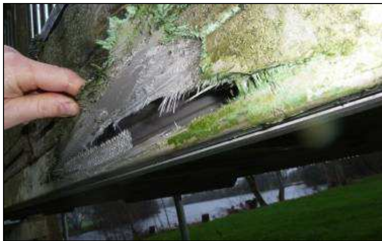
(b) Detail of the damage to the bottom 3-way component (December 2011)
