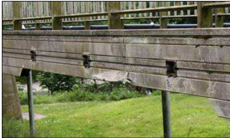
(a) Location of the damage (June 2008)
