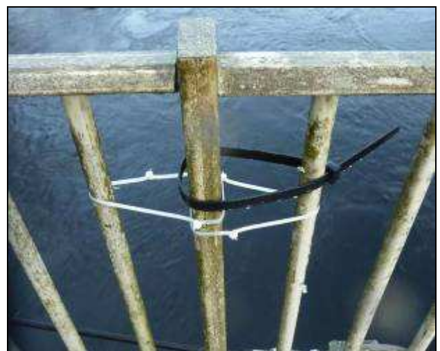
(b) Zip tie repair (December 2011)
