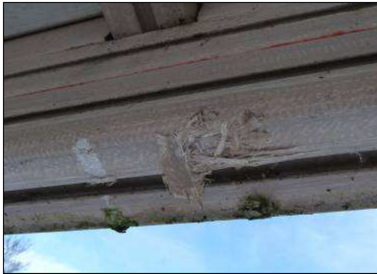
Figure 15. Impact damage to the underside of the deck (December 2010).
