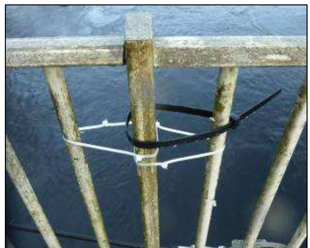
(b) Zip tie repair (December 2011)
